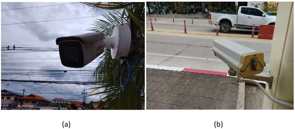
Fig. 2. The position of two installed CCTV cameras at the front gate of the university: (a) Camera 1 and (b) Camera 2.
